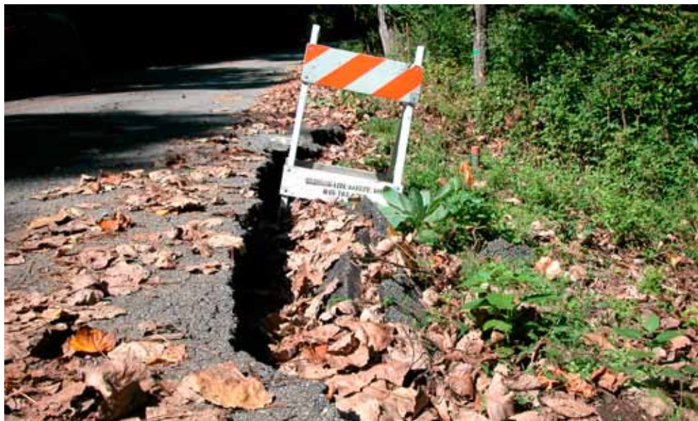
The landslide on Ridgewood Drive is scheduled for repair.
