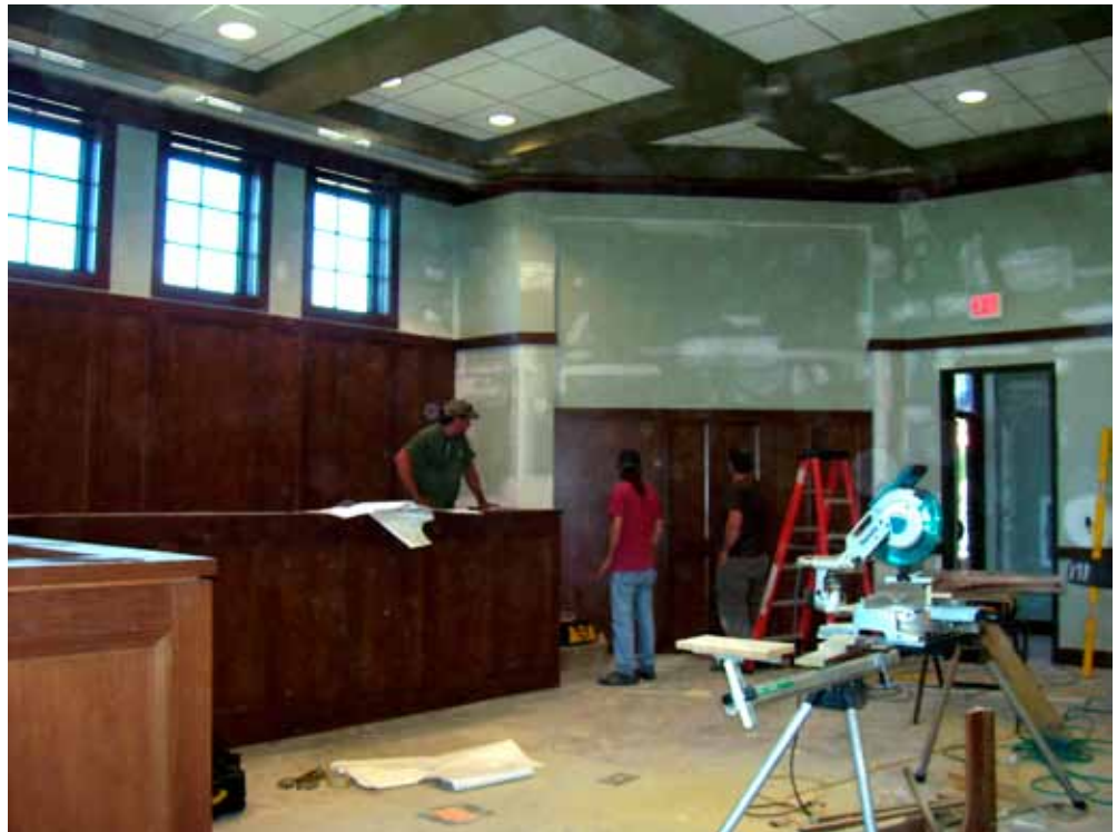
The new City Hall features a large meeting room and raised dais for board members.
